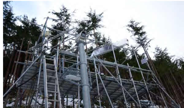
Figure 7. Audio system, Weatherproof digital camera and solar panels placed in Cyber Forest project site.
